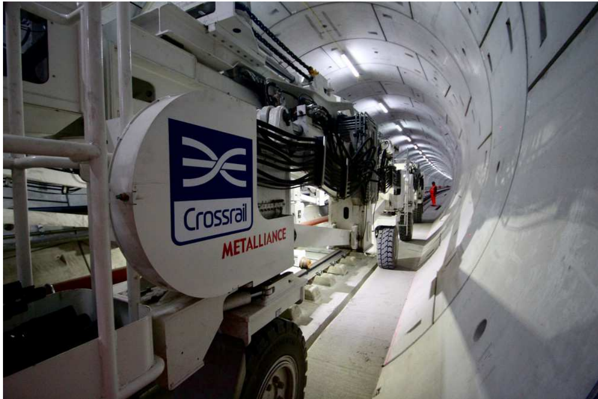
Multi-purpose gantry in use to install track in Crossrail Thames Tunnel (copyright Crossrail)
